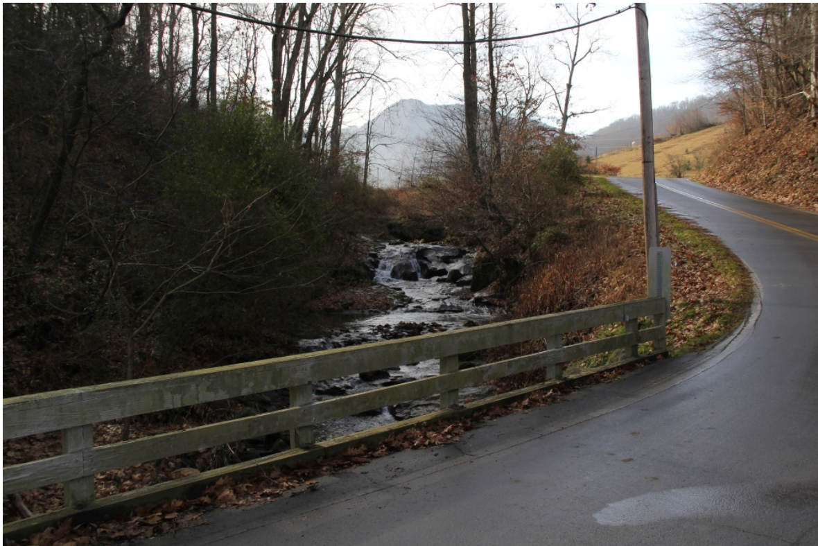
Bridge No. 371 on SR 1394 (Willow Creek Road) over Willow Creek, view to south
